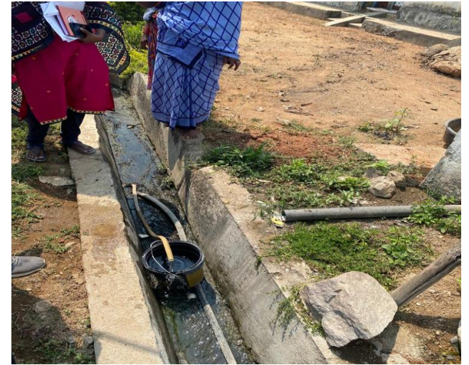
Secure pipeline connections
