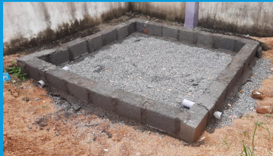
Rainwater harvesting unit.
